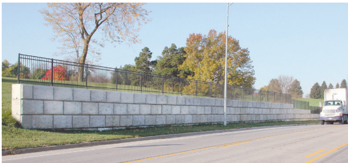
Just one of the beautiful new retaining walls with new fencing at the Harlan Cemetery.
